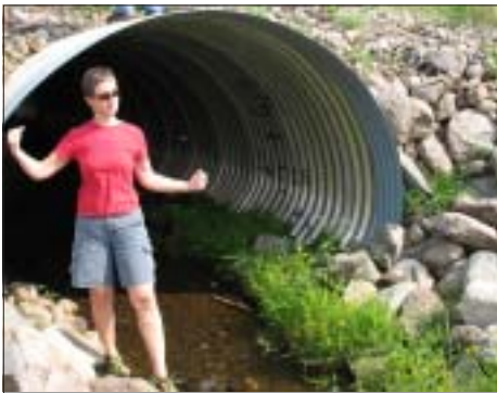
This culvert is sized to effectively handle a heavy rainfall drained from a large watershed.
